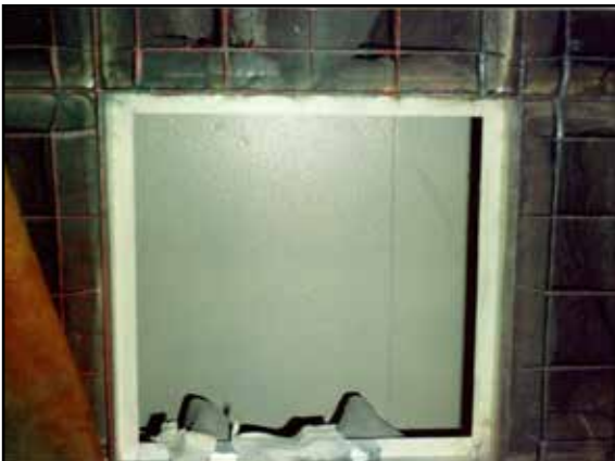
Clean Back Plenum
